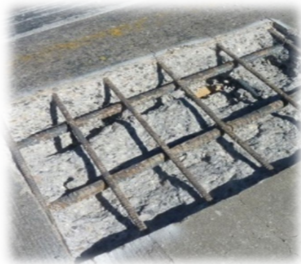
Deck Spall: Ideal Site Preparation
