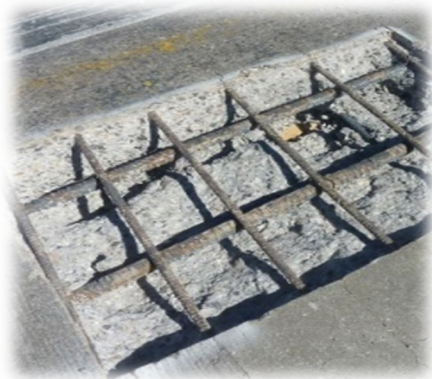
Deck Spall: Ideal Site Preparation
