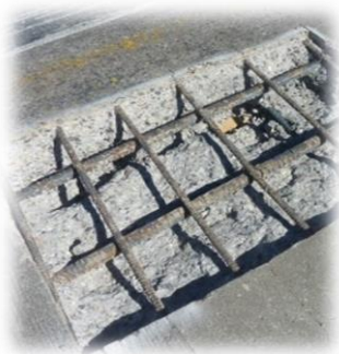
Deck Spall Ideal Site Preparation
