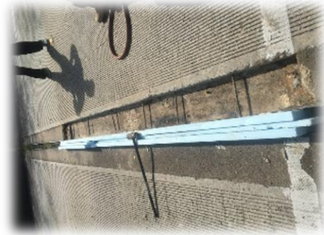
Use Foam Board to Establish Expansion Joints Use painter's tape with FTE
