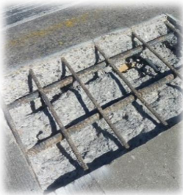
Deck Spall Ideal Site Preparation
